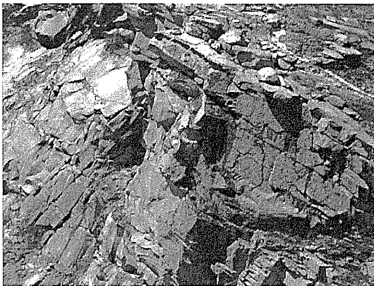
Figure 6. Post-collapse residual rock mass after the Profile toppled forward (left). Note broken steel turnbuckles on residual Forehead (topmost) slab and remnants of concrete water diversion trough at back.
