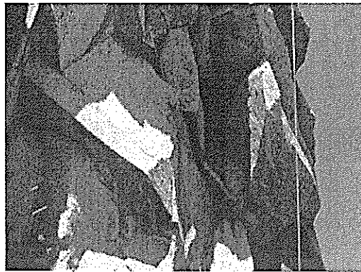
Figure 4. Close-up view of intersecting weathered joints in the pre-collapse rock mass. Chin block on right behind vertically hanging rope.
